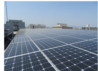
Solar power panels on a rooftop of the Kashima Office building
